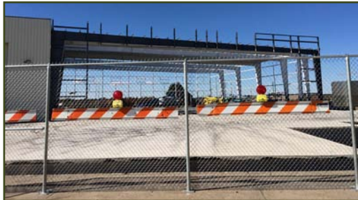
Construction of our 8th hangar on the Bismarck Airport has started! It is scheduled to be completed before 2016.
